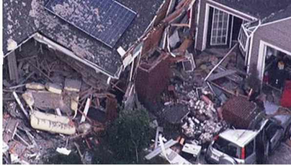
A home on Chickering Road in Lawrence exploded Sept. 13, 2018. The chimney crushed an SUV, killing Leonel Rondon. (WBZ-TV)
